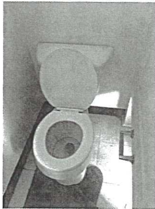
Men's room tank-type water closet
