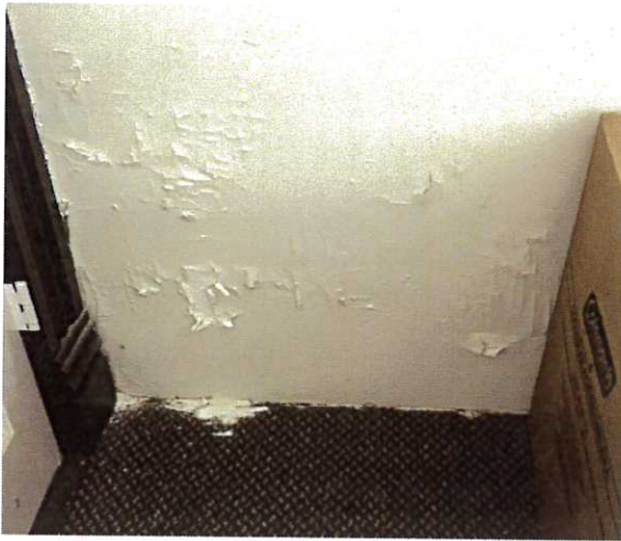
4.19 WALL DAMAGE FROM LEAKS
