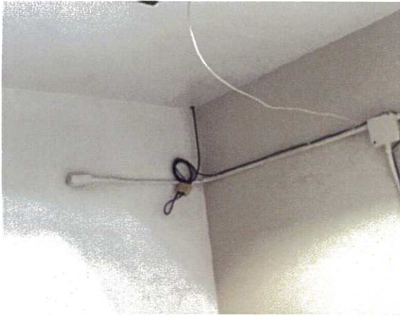
4.13 EXPOSED ELECTRICAL CONDUIT
