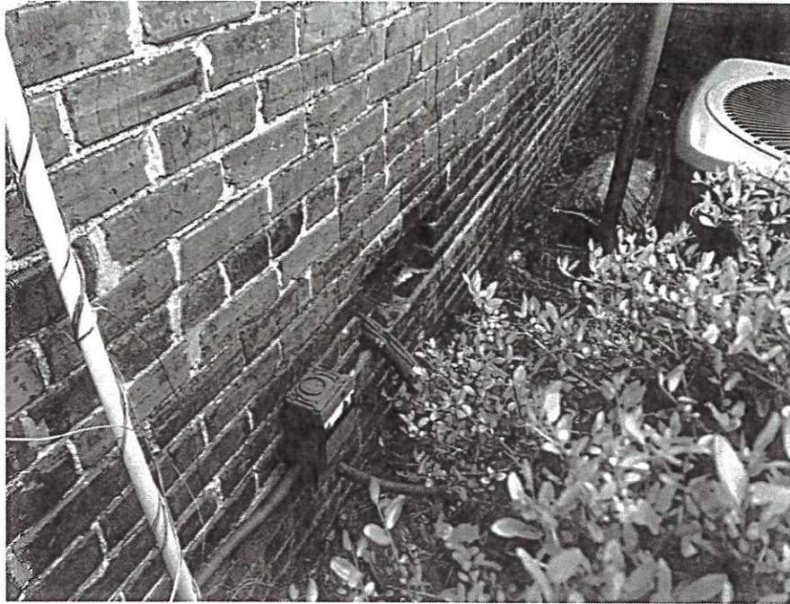
Picture No. 3 – Crawl Space Vent Where First Floor Framing was Observed
