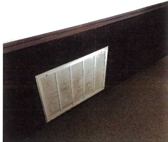
4.16 NON-COMPLIANT RETURN AIR IN HALL
