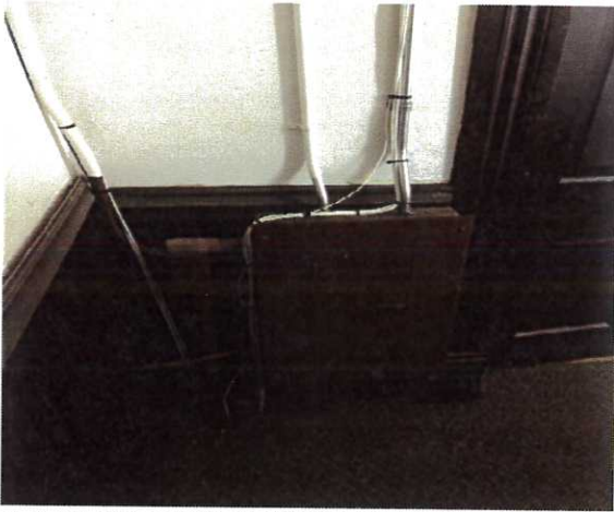
4.4.21 EXPOSED ELECTRICAL PANEL IN HALL
