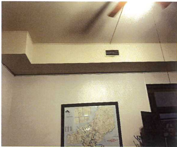
4.4.15 SECOND FLOOR EXPOSED HVAC DUCT
