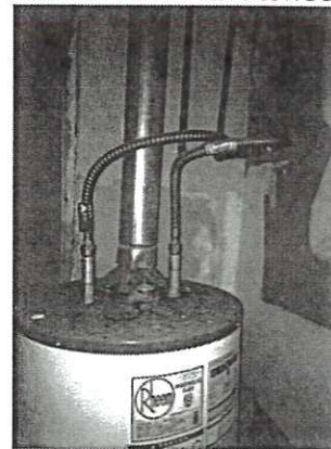
50 gallon natural gas water heater
