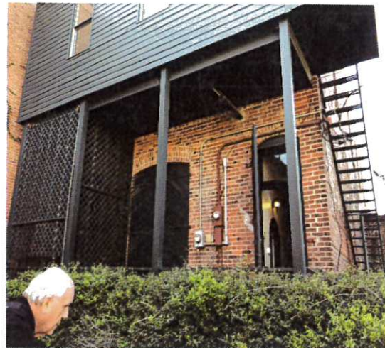
4.26 EXTERIOR MECHANICAL & ELECTRICAL
