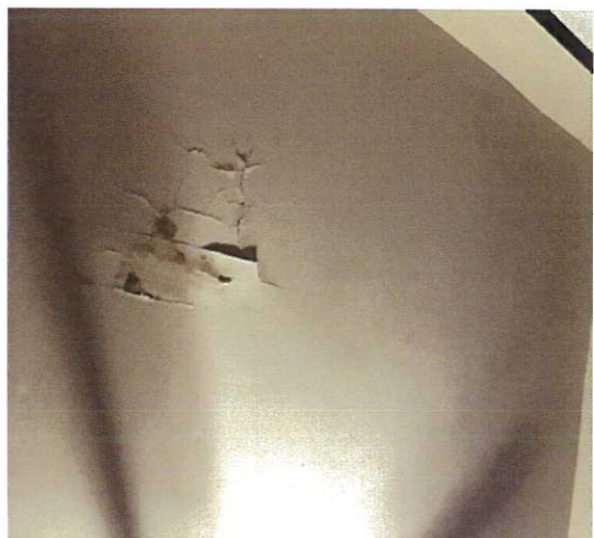
4.12 SECOND FLOOR CEILING LEAK
