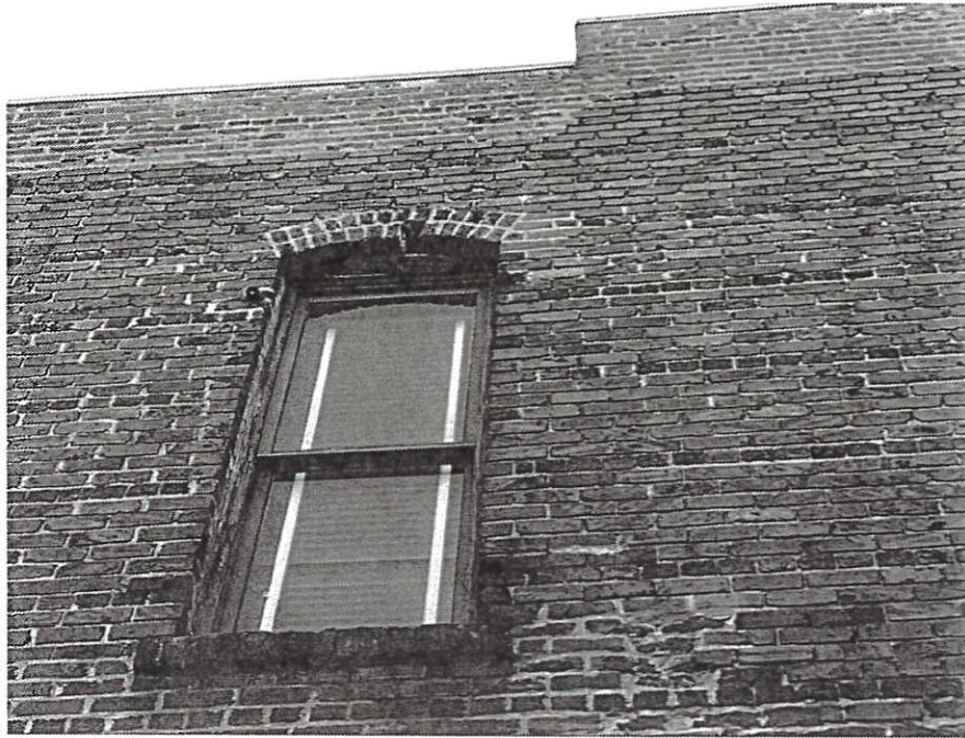
Picture No. 9 – Missing Brick in Arched Brick Lintel
