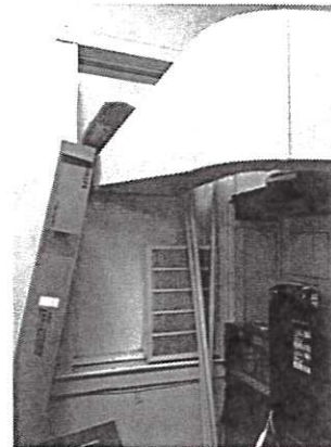
Supply and return duct at north wall
