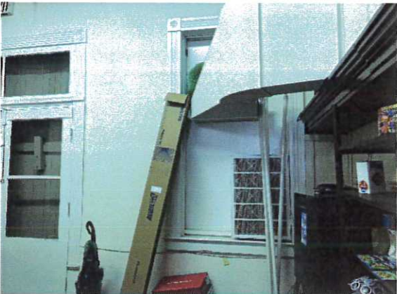
4.5 FIRST FLOOR EXPOSED HVAC DUCT
