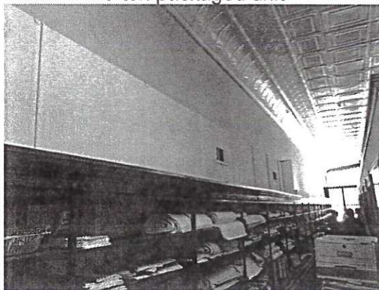
Supply duct along east wall
