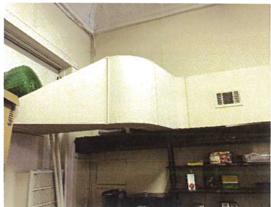
4.6 FIRST FLOOR HVAC EXPOSED DUCT
