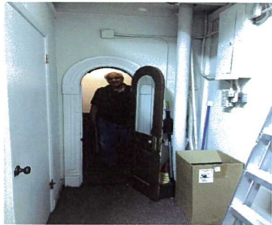
4.8 NON-COMPLIANT FIRST FLOOR DOOR
