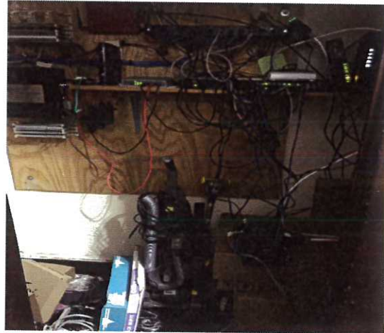
4.22 IT & ELECTRICAL CLOSET
