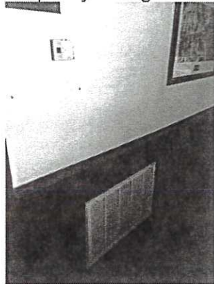
Return air grille and thermostat
