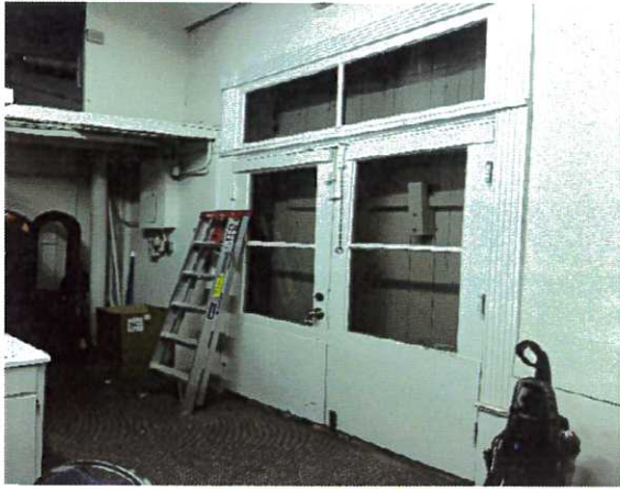
4.7 BLOCKED FIRST FLOOR EGRESS
